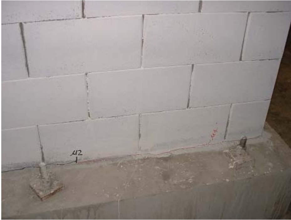
Figure 7-3 Base crack along total length of wall from both directions
