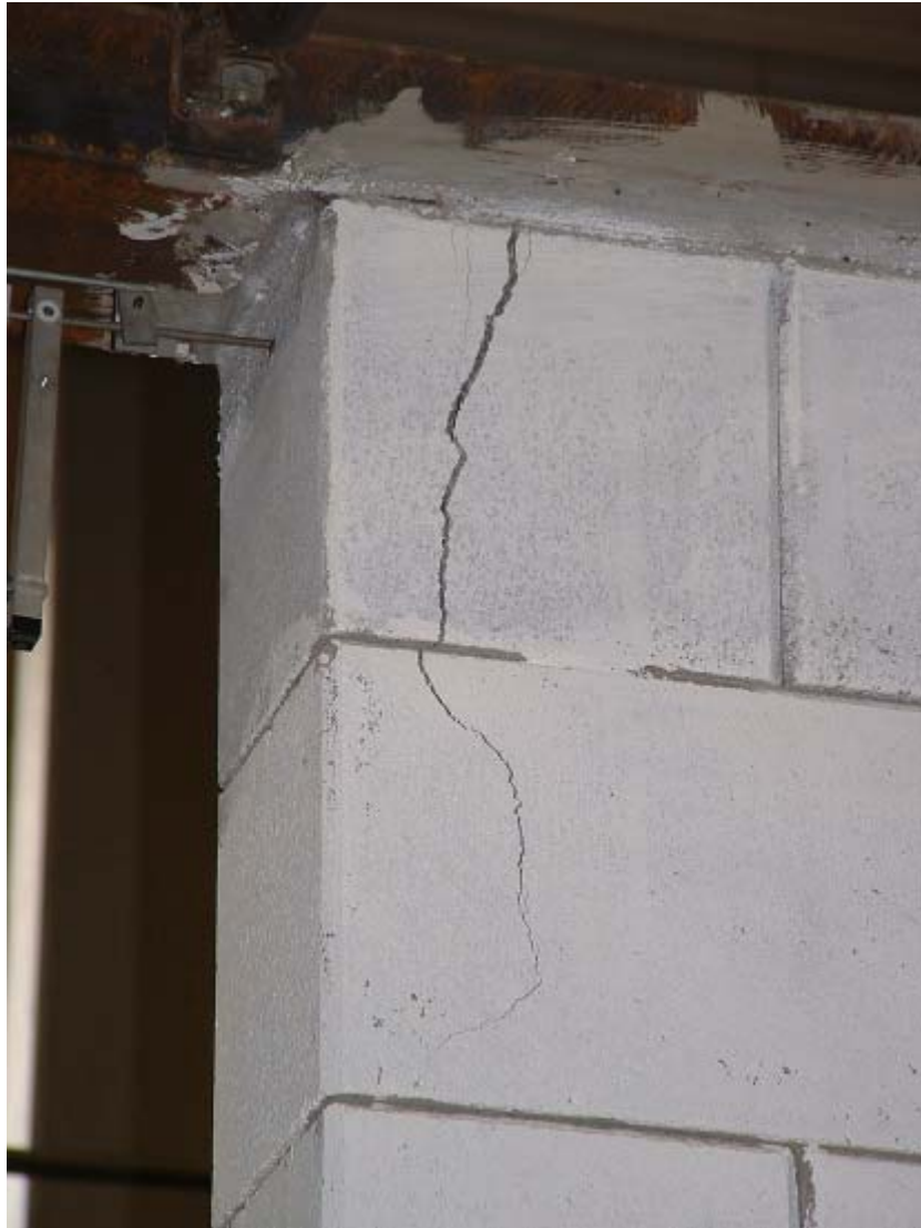
Figure 7-4 Crack at top corner now opened to 4 mm
