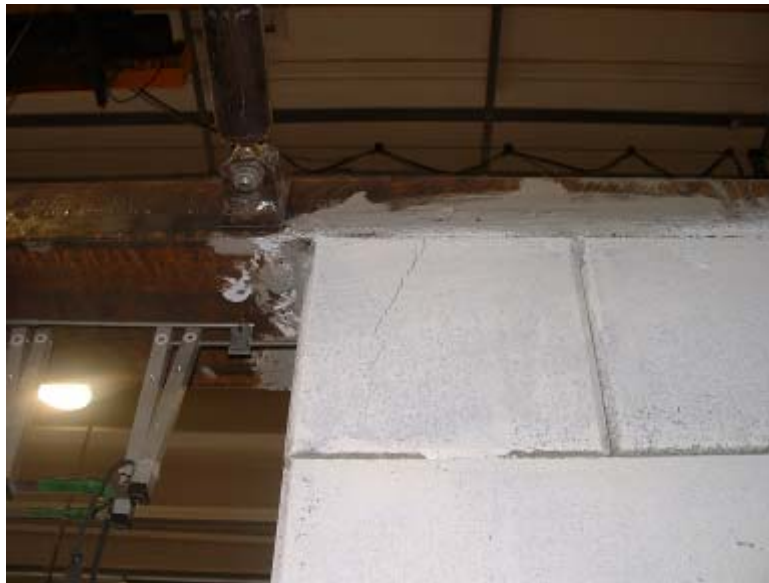
Figure 7-2 Crack at top corner on gauge end
